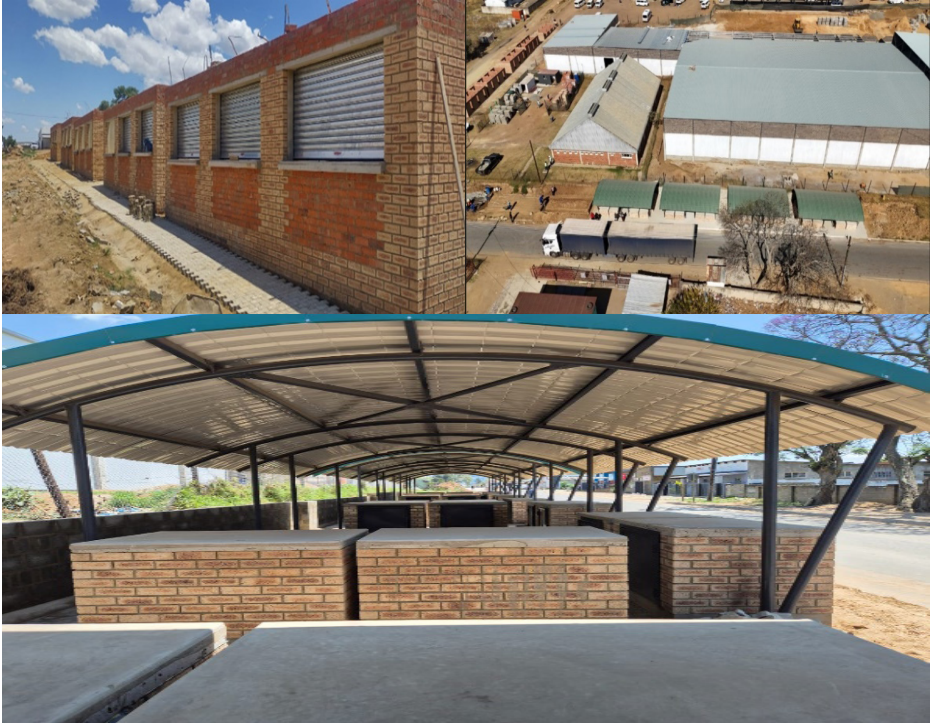
Figure 8.2.1: The below Close-range aerial view of open stalls (Green Roofs) with shelter. The closed stalls under construction are seen at the far left of the picture.
